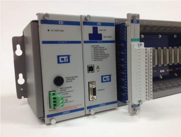
Figure 5 Physical Installation Picture
